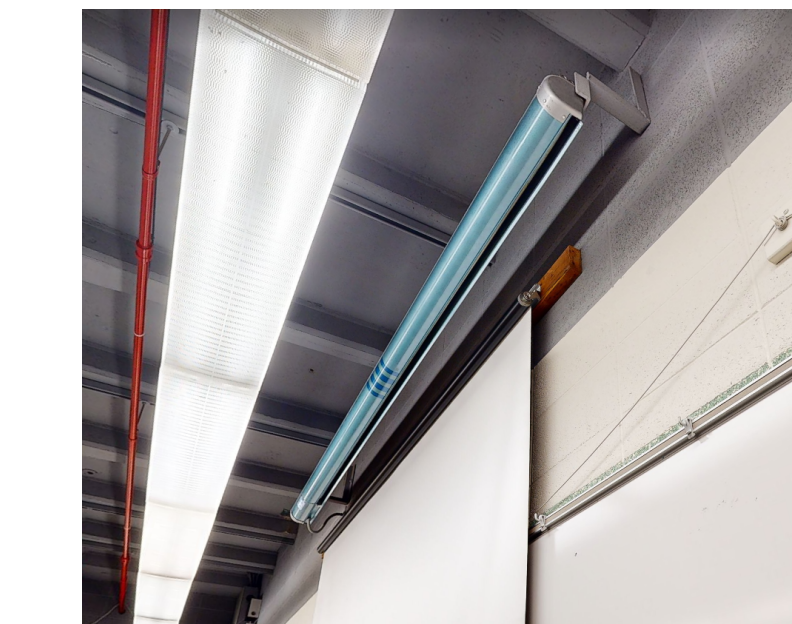
IMAGE 3 - EXAMPLE OF EXISTING PROJECTOR SCREEN AND BRACKETS.
